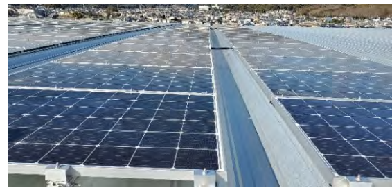
Solar power panels installed on the roof
